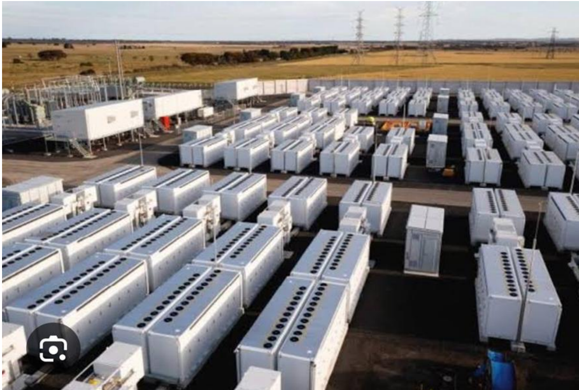
Figure 11 – Typical Battery Farm arrangement of 20 foot type containers.
