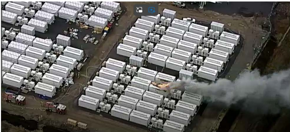
Figure 6: BESS Fire Incident in Victoria, 2021
